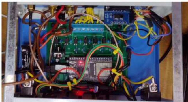
Figure 5 — The control unit interior.
