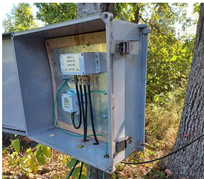
Figure 5 — The enclosure, cables, and ground connection. Note the drip loop on the antenna cable.
