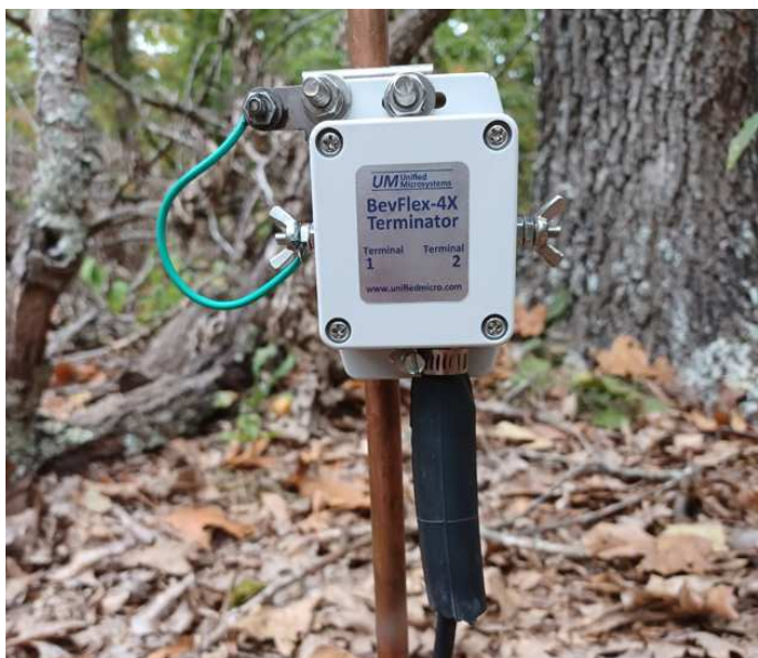
Figure 8 — The Terminator at the far end of the Beverage is mounted on a ground rod with the antenna cable attached.
