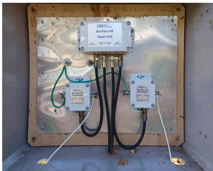
Figure 4 — The modules installed in the protective enclosure and connected to the white loop wires.
