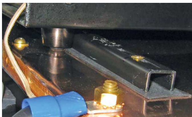
Figure 3 — Use a larger pilaster to keep large, heavy equipment in place on an inclined shelf. [Mark Kupferschmid, AC9PR, photo]
